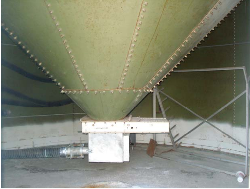
Interior View-Additional layer of steel inside silos that forms a cone at the bottom.
